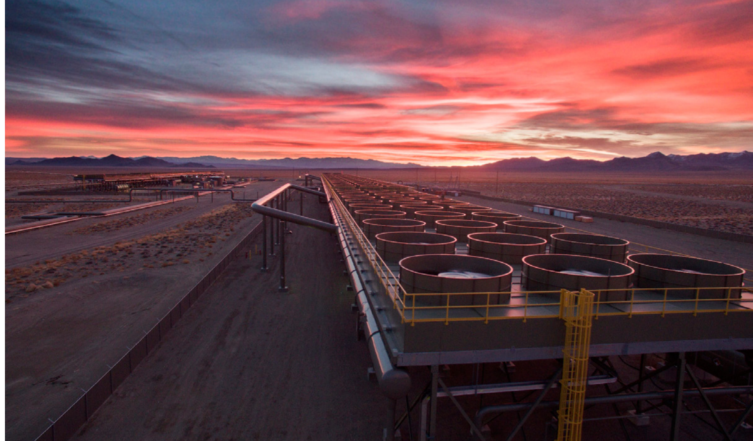
Don A. Campbell Complex, NV, U.S., 32 MW
